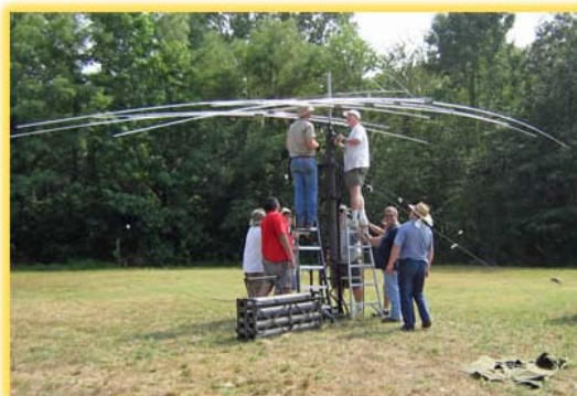
Force 12 C4S going up on AB-577 mast
